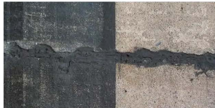
Even the expansion joint material has not been destroyed
